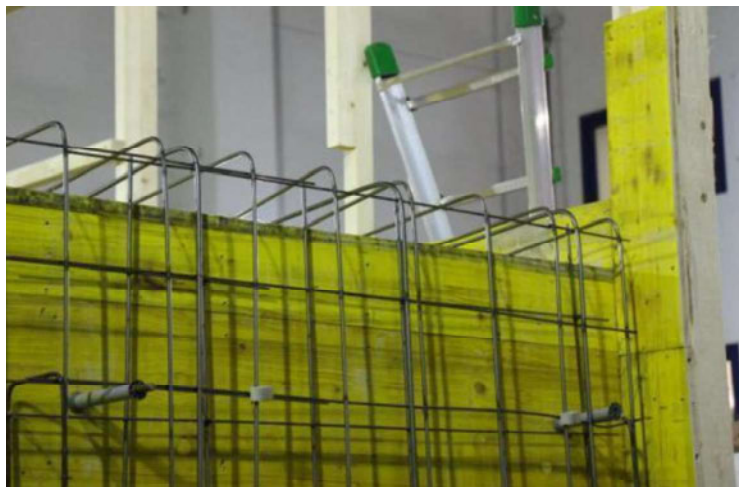
Figure A.8: Detail of the in-floor bent rebars placed in a wall-slab joint of the EUC-BUILD-3 specimen (adapted from [Brunesi et al, 2017]).
